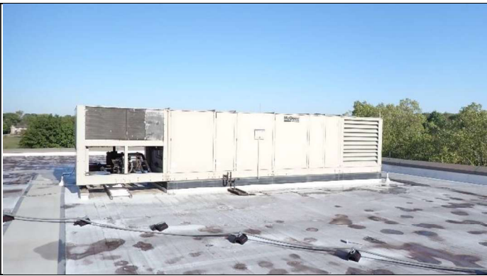
Overview of RTU
