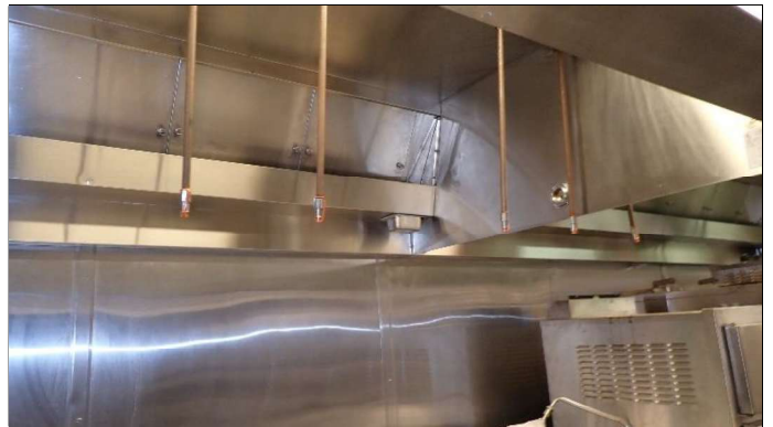
Cooking range suppression nozzles
