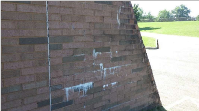
Typical efflorescence on brick surface
