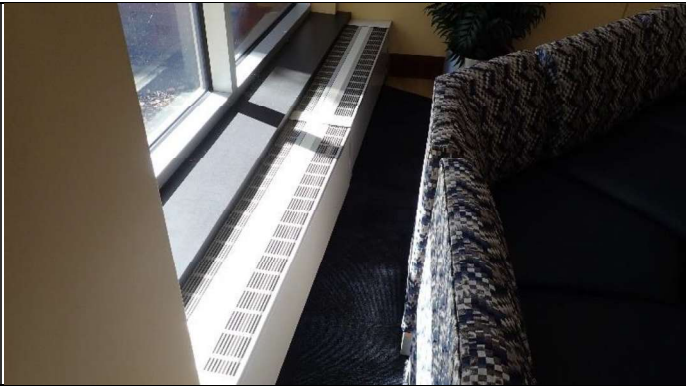
Overview of radiator
