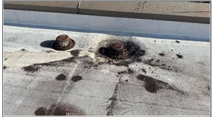
Internal roof drain
