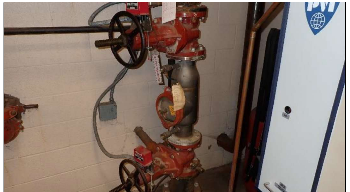
Backflow prevention valve
