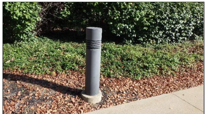
Overview of exterior light fixture
