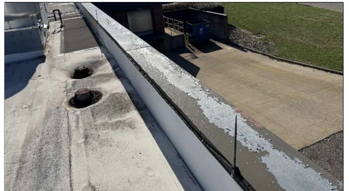
Deteriorated finish on metal coping
