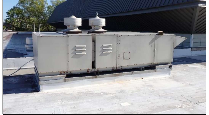
Industrial heater with make-up air
