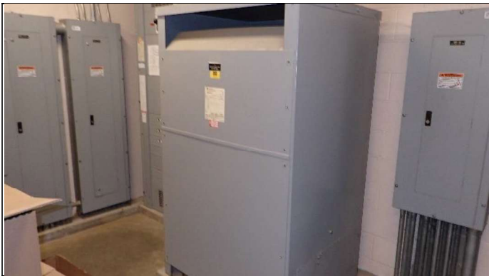
Electrical distribution equipment
