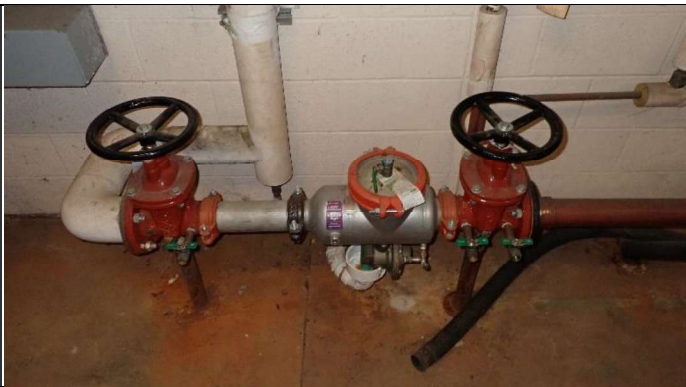
Water service entrance and backflow prevention valve
