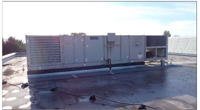
Overview of RTU
