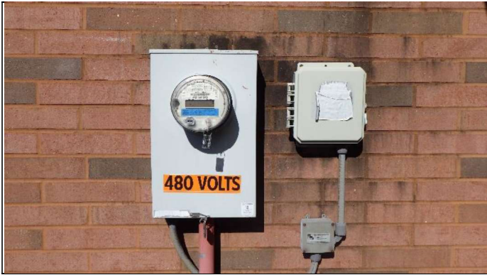
Electrical service meter
