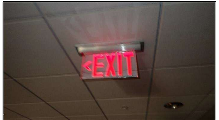
Illuminated exit sign
