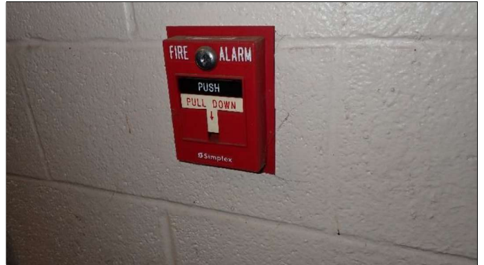
Typical pull-down station
