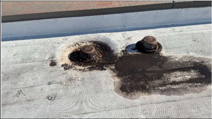
Internal roof drain
