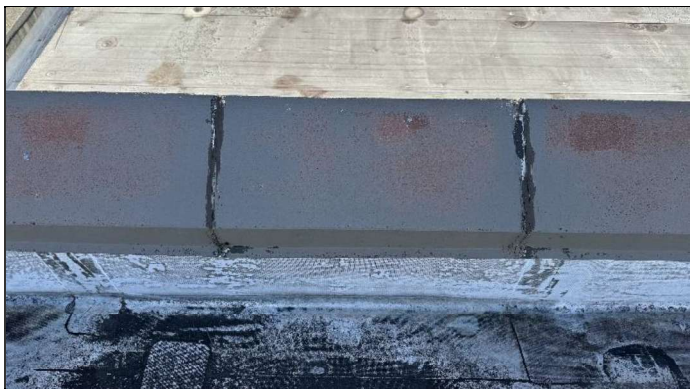
Deterioration of metal coping joints
