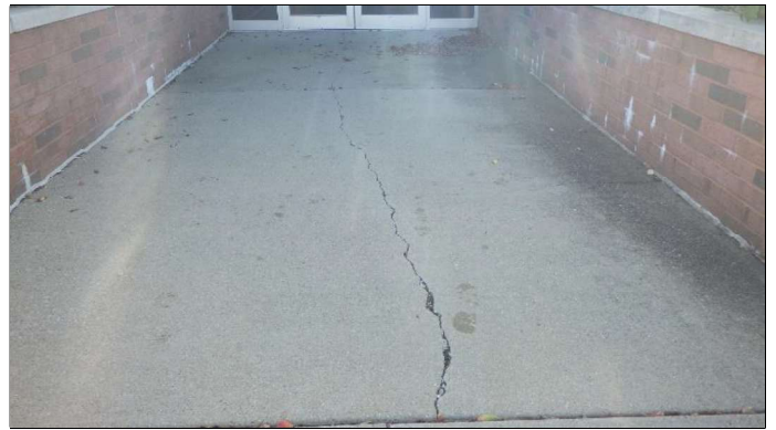
Concrete sidewalk crack
