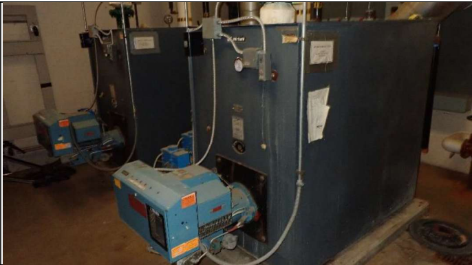
Overview of boilers
