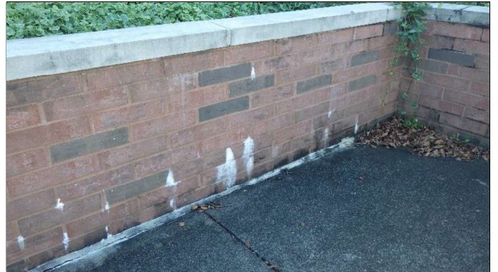
Typical efflorescence on brick surface
