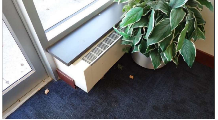
Overview of radiator
