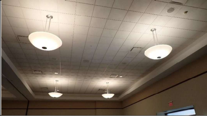
Overview of interior light fixtures
