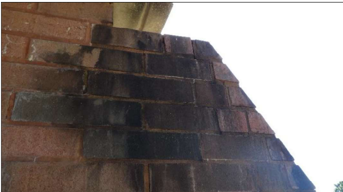
Typical stains on brick surface
