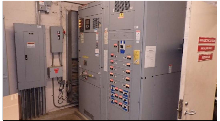
Electrical distribution equipment
