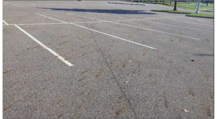
Asphalt pavement crack
