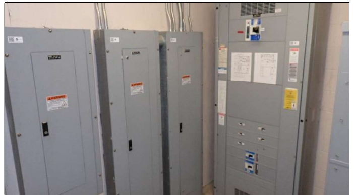
Electrical distribution equipment
