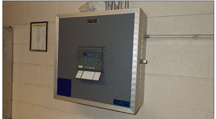
Boiler control panel
