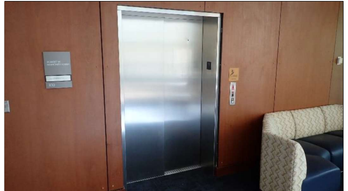
Overview of traction elevator
