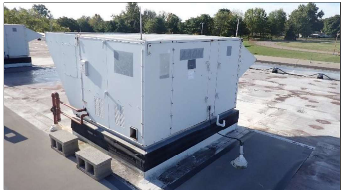
Overview of RTU
