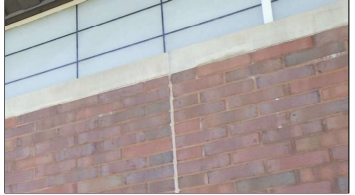
Typical deteriorated sealant in vertical joint
