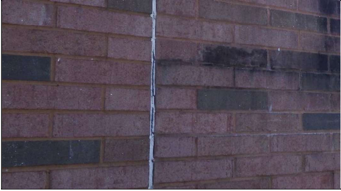
Typical deteriorated sealant in vertical joint
