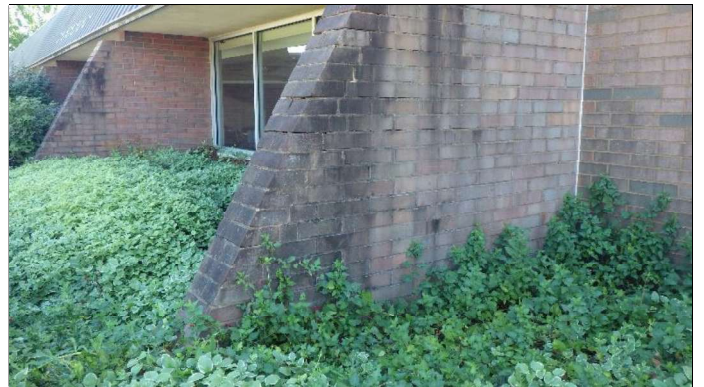
Typical stains on brick surface
