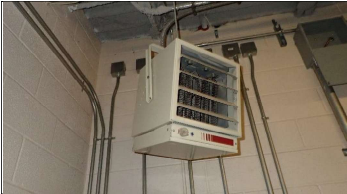
Electrical unit heater
