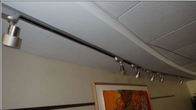
Overview of interior light fixtures
