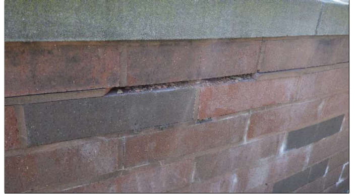
Typical mortar cracks
