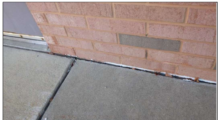
Typical deteriorated base sealant to brick veneer
