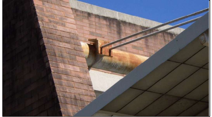
Typical stains on steel framing
