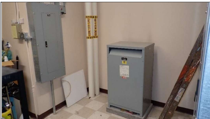
Electrical distribution equipment
