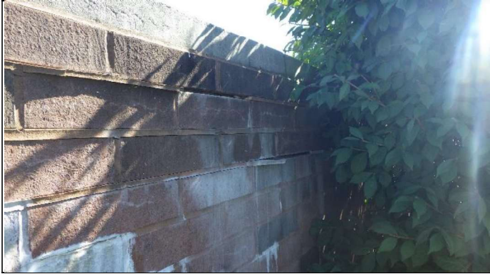
Typical mortar cracks
