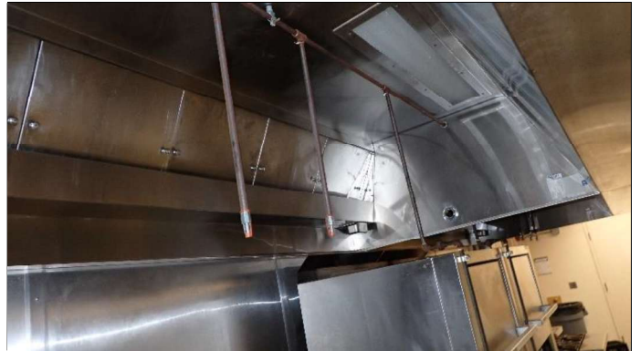
Cooking range suppression nozzles
