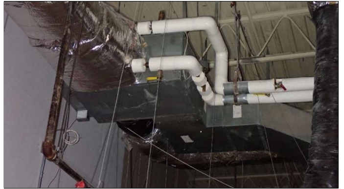
Overview of terminal unit
