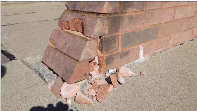
Cracks in the brick veneer
