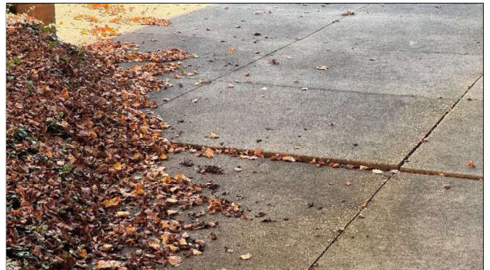
Potential tripping hazard in walkway
