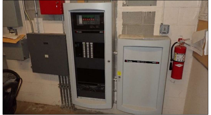
Fire alarm control panel
