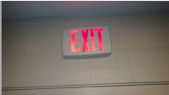
Illuminated exit sign
