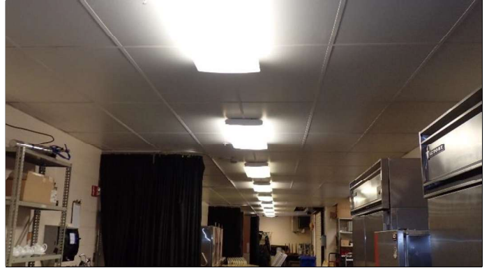
Overview of interior light fixtures
