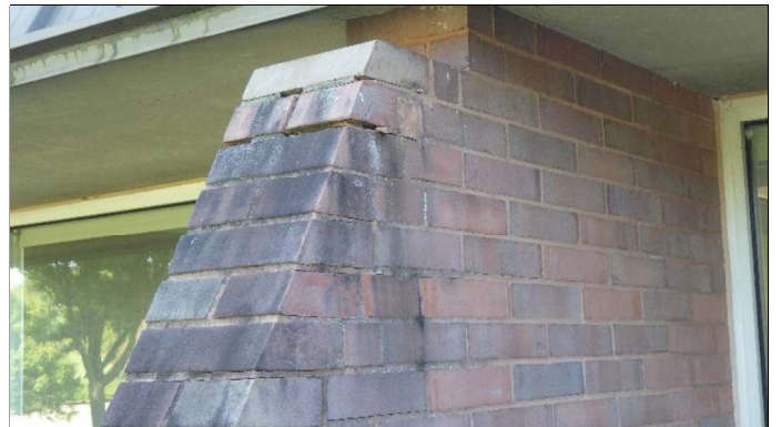
Typical mortar cracks
