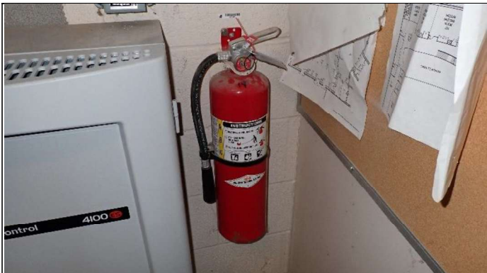
Dry chemical fire extinguisher
