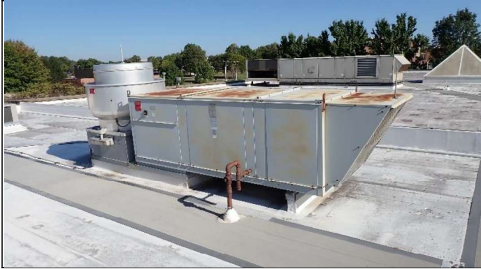
Industrial heater with make-up air
