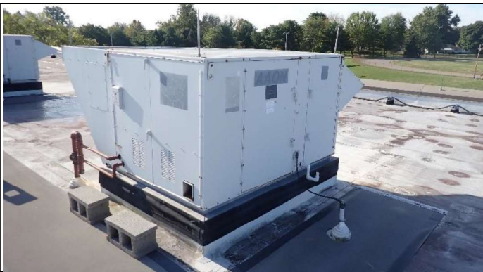
Overview of RTU
