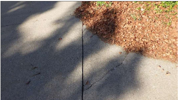
Concrete sidewalk crack
