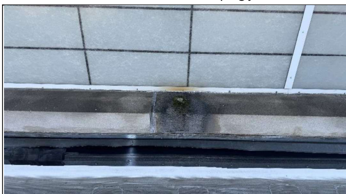
Deterioration of limestone coping above dining area
