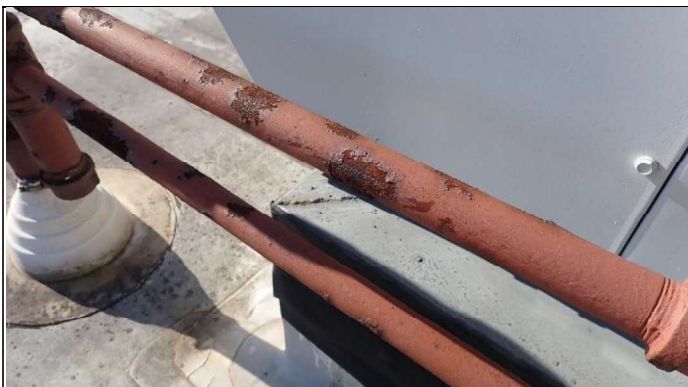
Surface corrosion on natural gas distribution pipes
