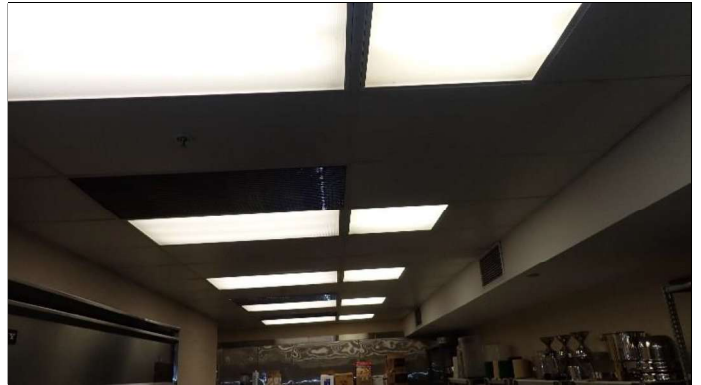
Overview of interior light fixtures
