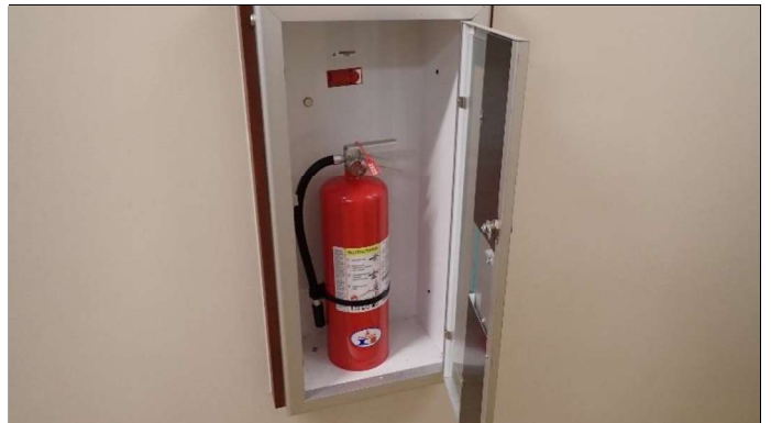
Dry chemical fire extinguisher
